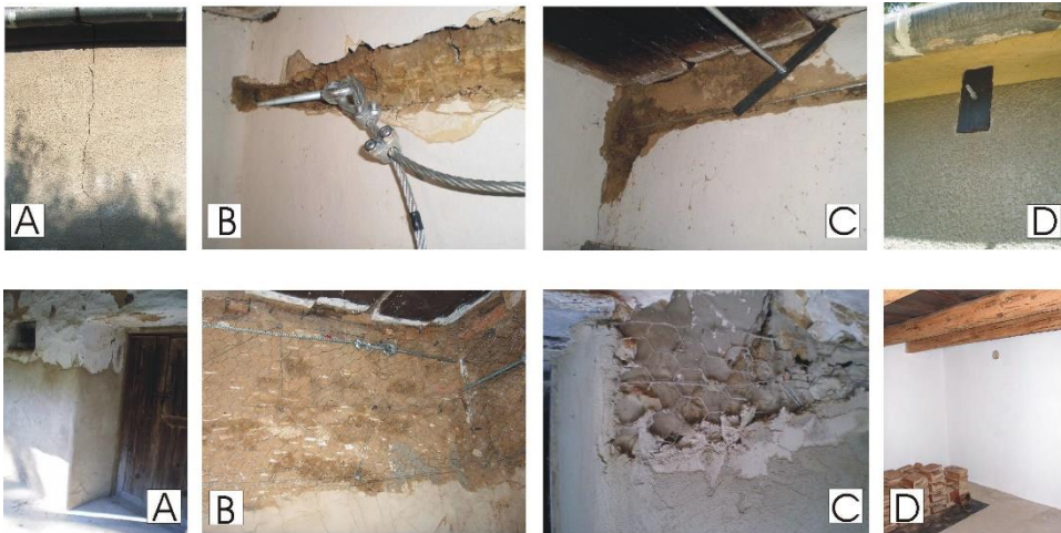
Figure 8, 9. Two renovation processes of the adobe house. Upper part: strengthening of the of the walling: (A) splitting (B) connection of the cable-rope to the screw (C) The stretched cable-rope in inside (D) The screw with underlay in outside. Lower part: Strengthening of the surfaca: (A) the moulding surface in outside (B) the wire mesh mounted on the wall (C) rough-casting (D) polished plastering in inside. (Source: Experimental work by the author Á.N.)
