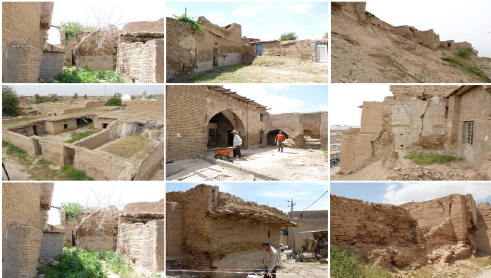
Partially collapsed structures
