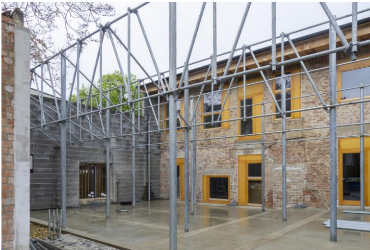
Figure 3 Drying workshop, under construction - refurbishment of the old workshop building. Department of Architecture UD. Photo: Tamás Szentirmai
